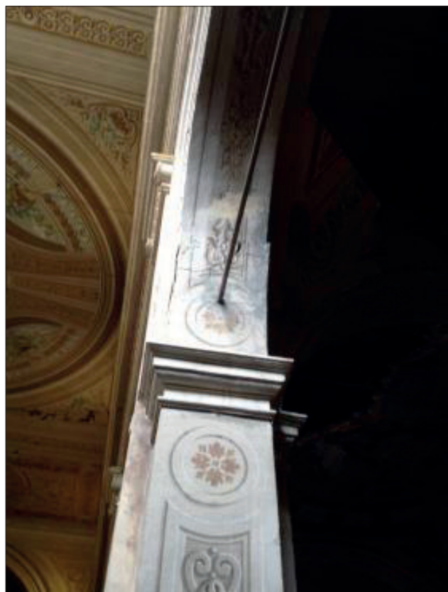
FIGURE 14 Crack and translation on the arch
