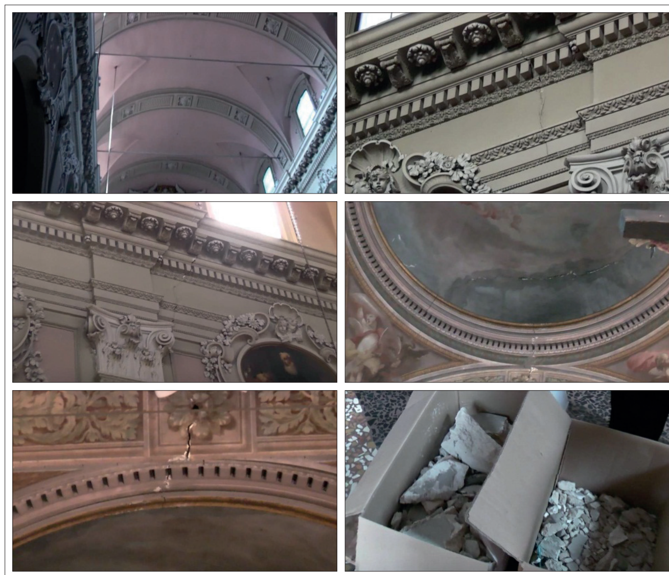
FIGURE 32 Damage to the Church of San Lorenzo (Budrio, Bologna)
