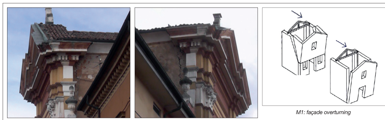
FIGURE 10 Cento (Ferrara) historic centre: the church of San Filippo Neri and main collapse mechanisms
