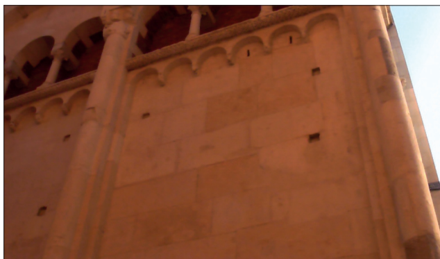
FIGURE 24 The San Geminiano Cathedral: potential overturning of the façade
