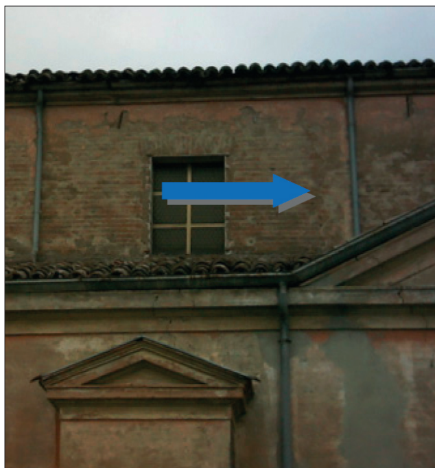
FIGURE 9 Passing through vertical crack
