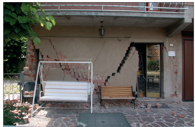
FIGURE 13 Serious failure of the walls, the damage is grade 4
