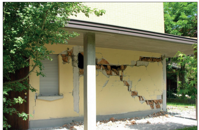
FIGURE 17 Damage to ground floor wall
