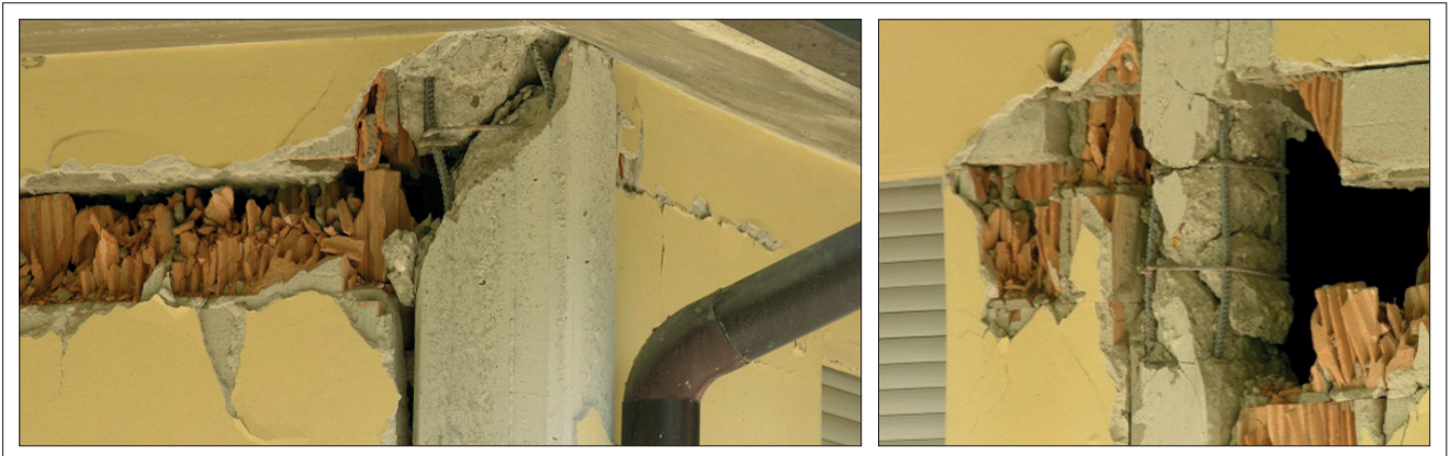
FIGURES 18-19 Failure of RC columns
