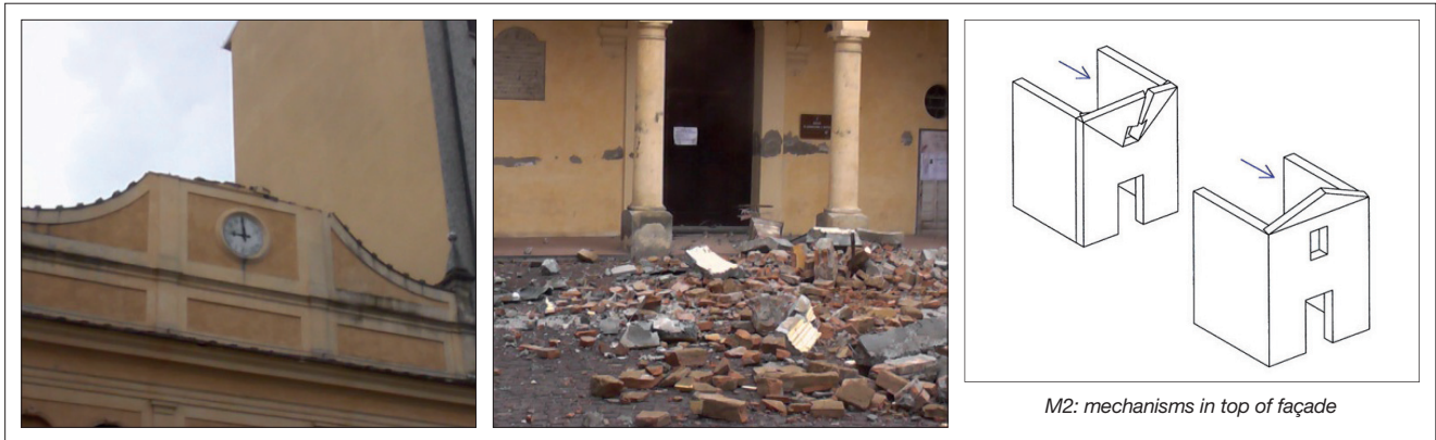
FIGURE 11 Cento (Ferrara) historic centre: the Church of San Sebastiano and San Rocco (Convent of Friars Capuchins) and main collapse mechanisms
