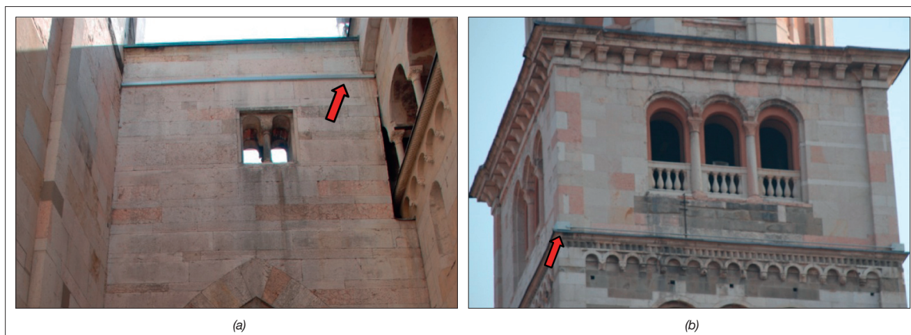
FIGURE 22 Monitoring and seismic devices: relative displacement measure device between Cathedral and Tower (left); b) steel tie all around the last square level of the Tower (right)
