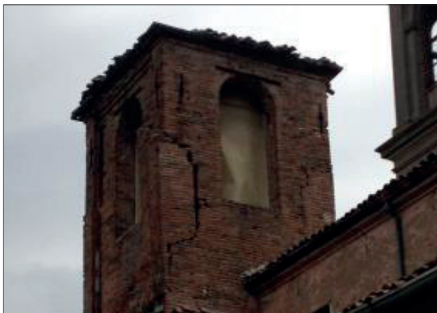
FIGURE 15 Separation and expulsion of the corner
