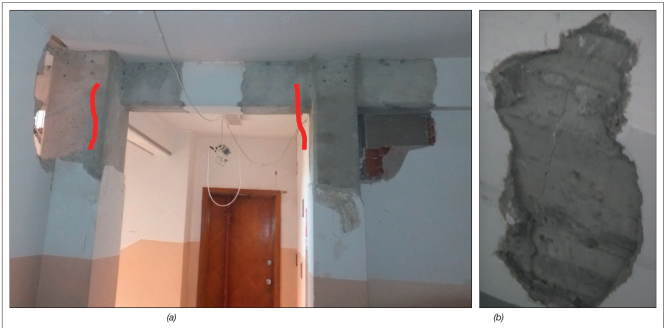
FIGURE 32 Structural seismic damage: a) location of the cracks on the stair beams; b) crack detail
