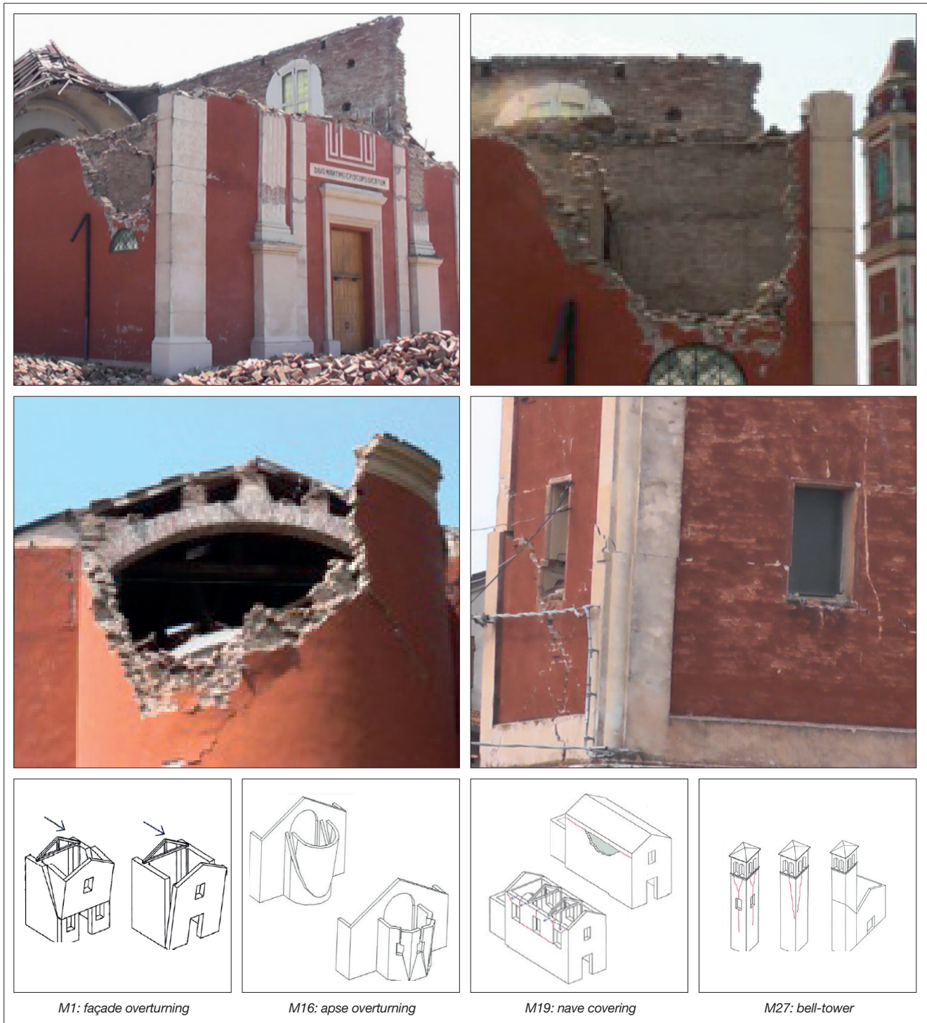
FIGURE 5 Damage in the San Martino di Tours church and bell-tower in Buonacompra (Cento, Ferrara) and main collapse mechanisms
