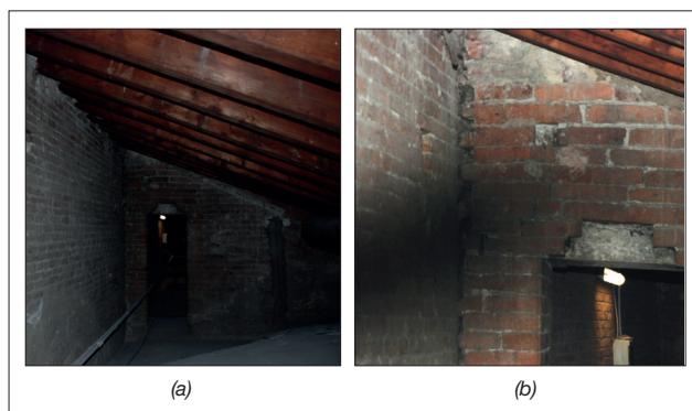
FIGURE 25 The San Geminiano Cathedral: overturning of the lateral transversal walls
