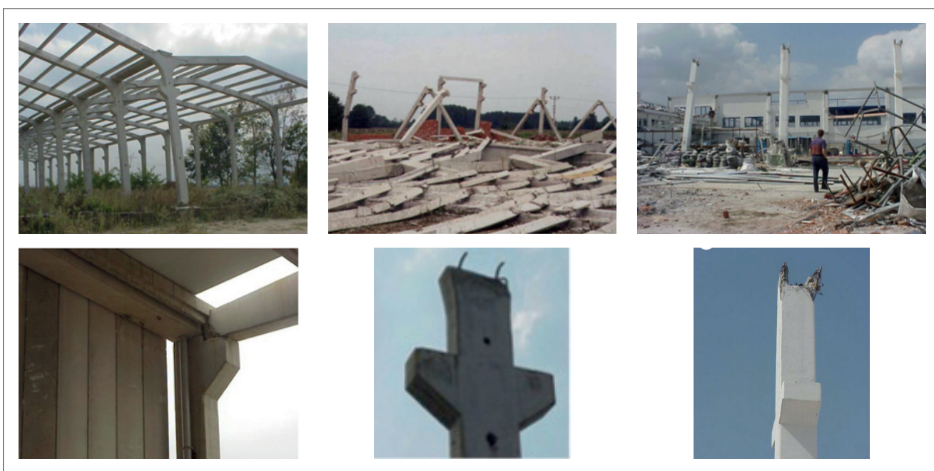
FIGURE 17 P/p. r.c. structures, with different stages of construction and seismic behaviour, located in the epicenter area of the Kocaeli earthquake, and details of the connections [11-14]
