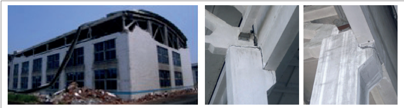
FIGURE 18 Damage and partial collapse of the Xiting Package Ltd. Factory complex in Mianzhu City, Wenchuan, China [15]
