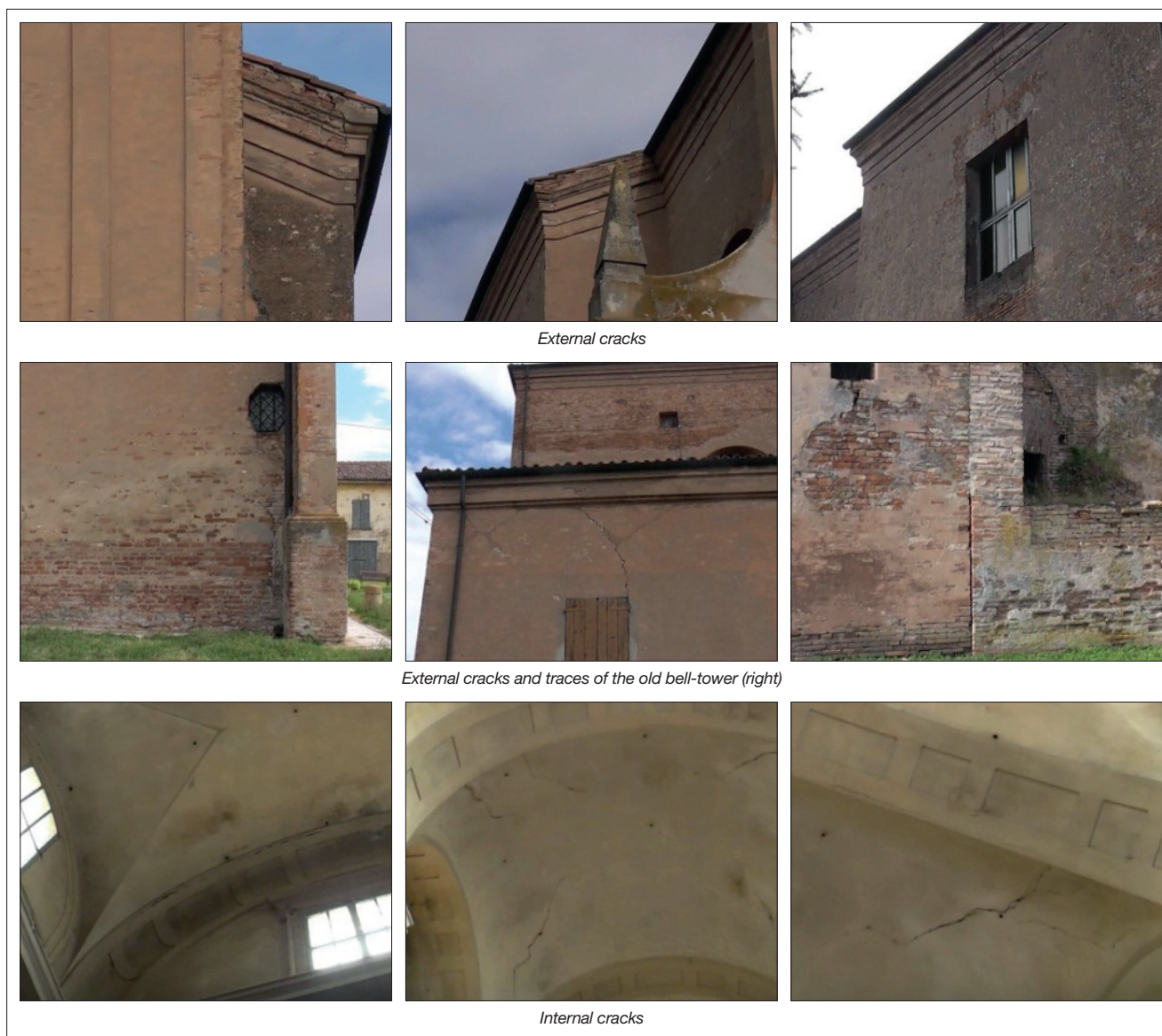
FIGURE 29 Damage mechanisms in the Ghirlandina Tower (Modena)
