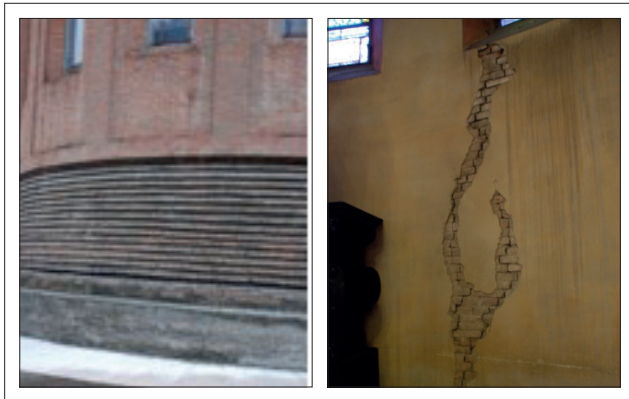
FIGURE 16 Subsidence phenomena: a) external view; b) internal view
