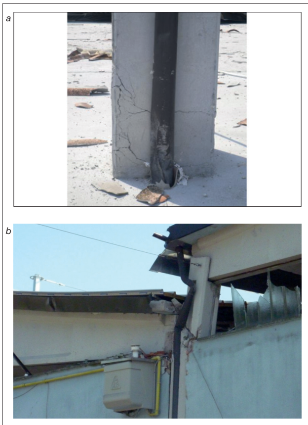
FIGURE 11 Damage to columns Source: ENEA
