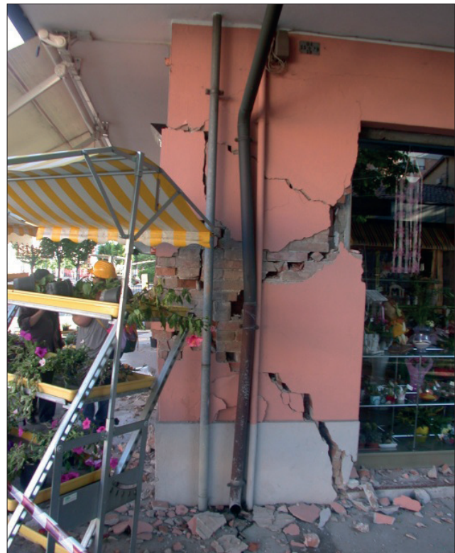
FIGURE 8 Heavy diagonal cracks with partial loss of connection between external walls (damage of grade 4)
