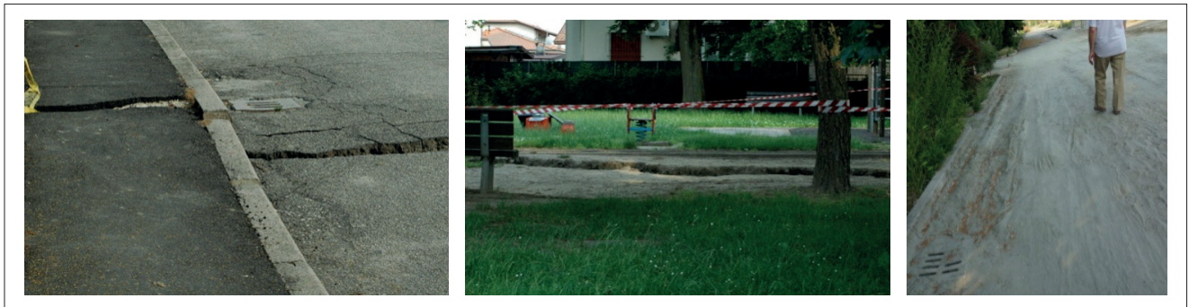
FIGURE 10 Sant'Agostino Municipality: one of the most damaged town by the earthquake of May 20 th
