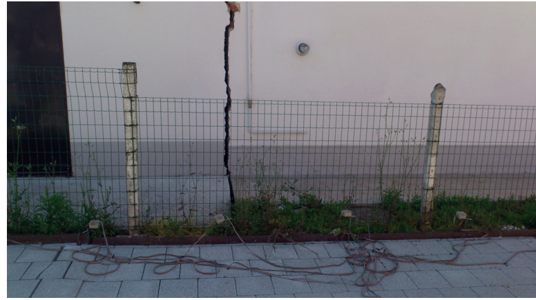
FIGURE 3 Side view of the investigated building with structural damage. The residential building is situated in Via Argine Postale, 57, Mirabello village (Italy). Near the fence, the seismic cables with geophones can be seen
