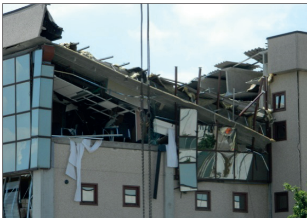
FIGURE 7 Longitudinal slipping of the roof beams Source: ENEA
