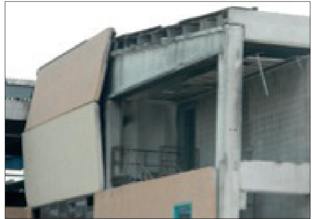
FIGURE 13 Detachment of the external wall Source: ENEA
