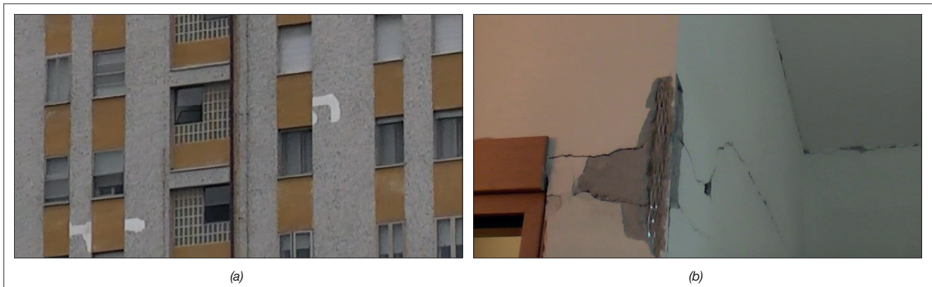
FIGURE 33 Non-structural seismic damages: a) façade covering layers; b) partition walls
