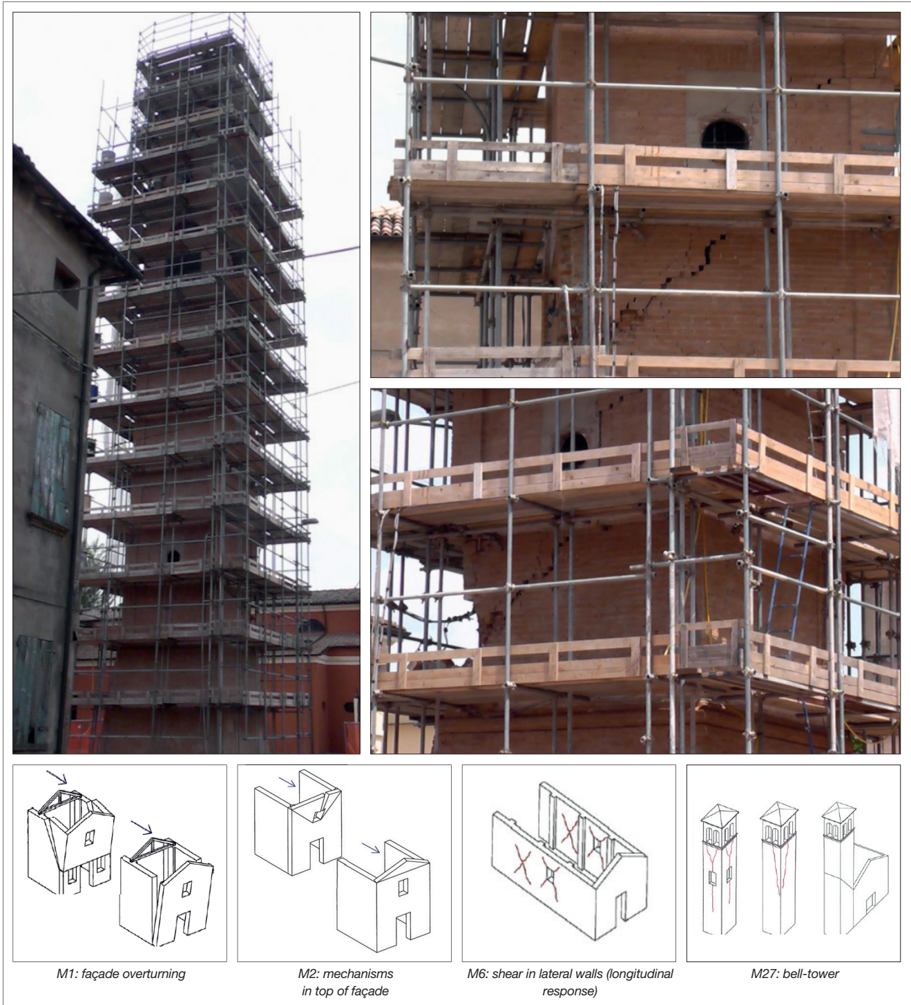
FIGURE 8 Damage to the Sant'Anna church in Reno Centese (Cento, Ferrara) and main collapse mechanisms
