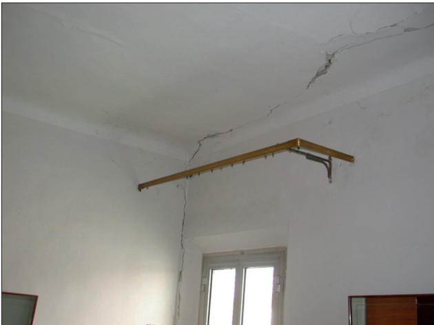
FIGURE 10 Bondeno: damage of grade 2-3 (EMS98 classification) Source: ENEA
