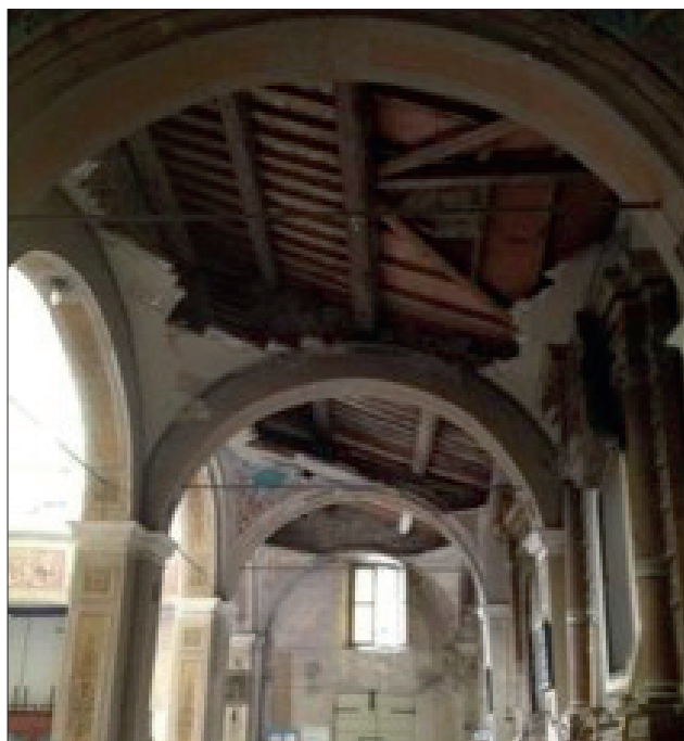
FIGURE 5 The collapsed vaults of the left nave
