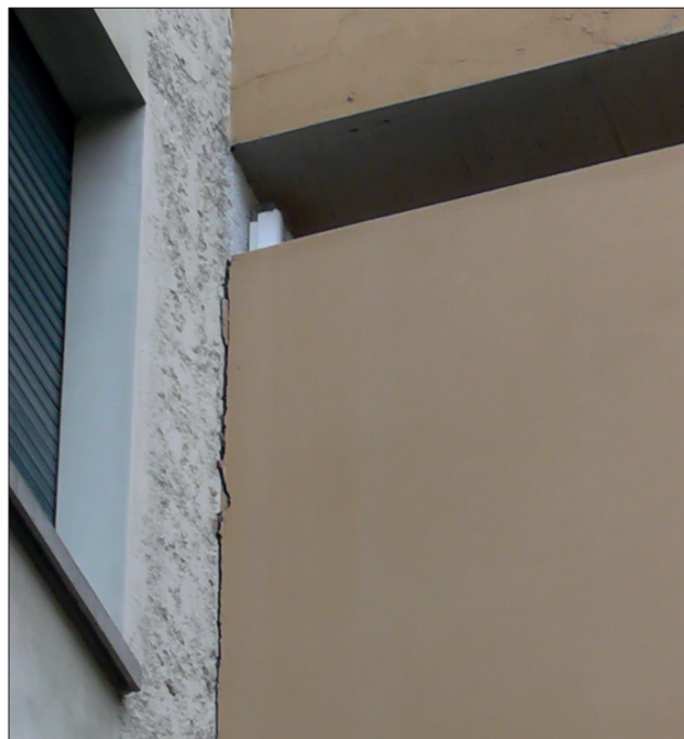
FIGURE 27 Detachment of the parapet of some balconies
