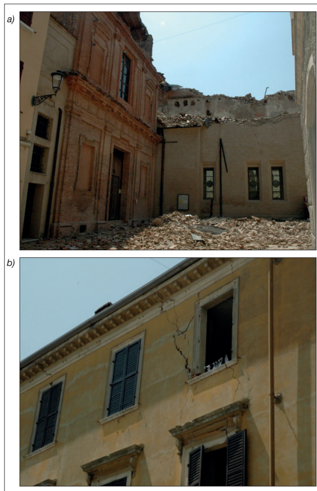
FIGURE 12 Mirandola. Damage in the historical downtown Source: ENEA
