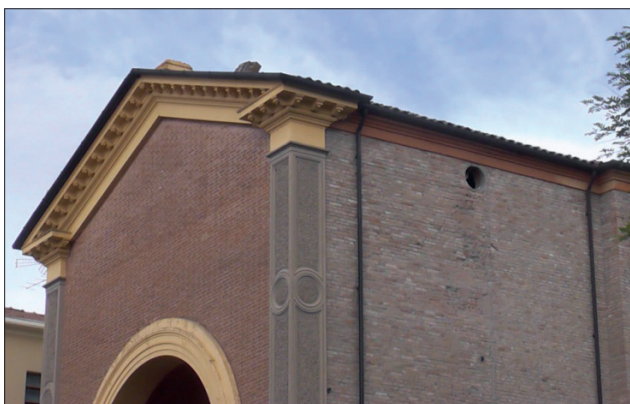
FIGURE 13 Cento (Ferrara) historic centre: the Church of San Pietro and main collapse mechanisms (middle above)
