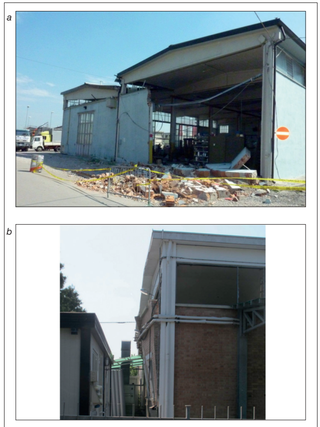
FIGURE 14 Solid brick cladding damage Source: ENEA
