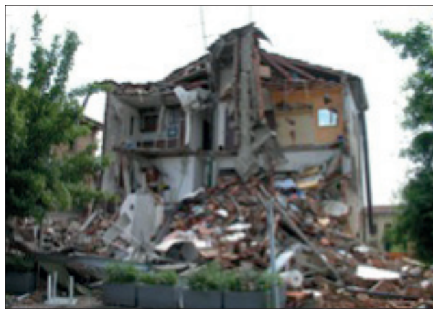
FIGURE 4 The front part of the building has completely collapsed; the damage grade is 5
