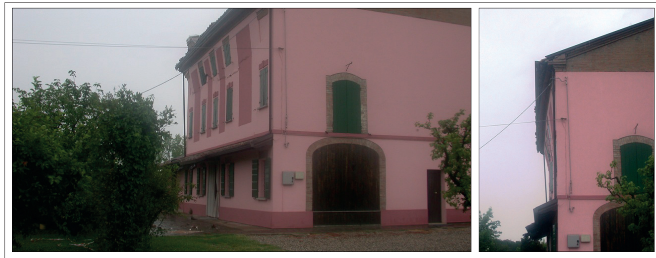
FIGURES 9-10 Out-of-plane mechanism of the upper part of the longitudinal façade
